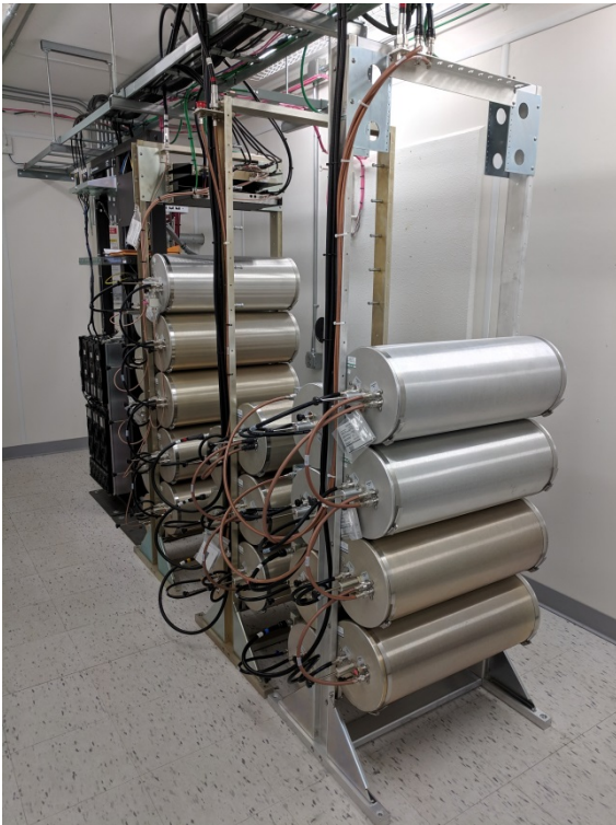
Figure 7 - Combiner system on Mansface to allow new repeaters to use existing antennas on the tower
