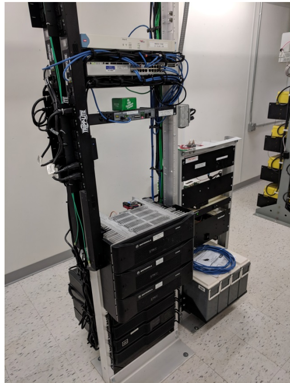
Figure 6 - New repeaters installed in the rack along with paging radio
